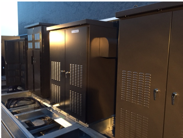
Large-Sized Electricity Storage System
